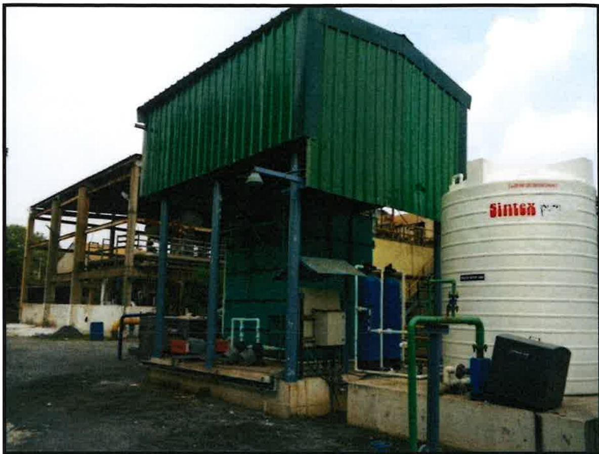
Photograph of STP commissioned at Plant - II
